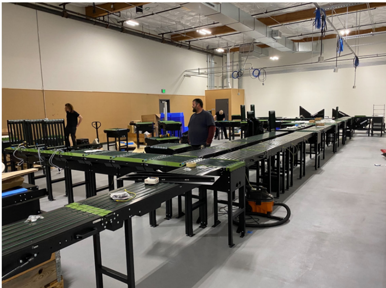
The new AMHS in action at the Maintenance and Operations Center
